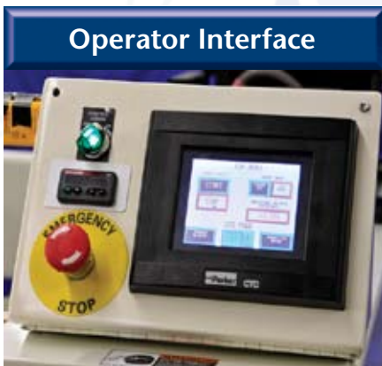
Operator interface with color monitor and PLC controlled sequence of operation.
